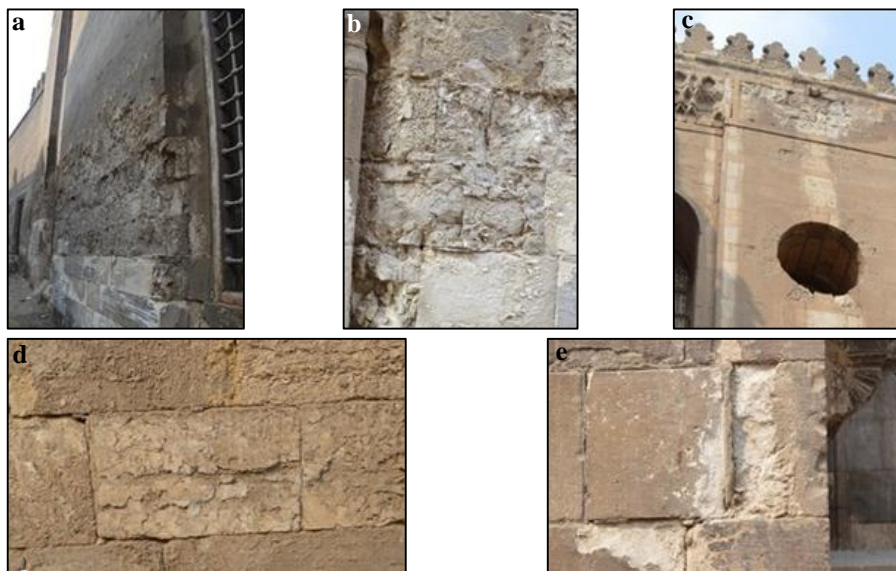
Figure (3) Shows weathering phenomena of the limestone used in Qaytbay mosque a. b. lower parts, c. upper parts, d. and e. middle parts of the mosque walls
